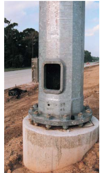
Shown here is the area the RKI winch is installed in the light pole.
